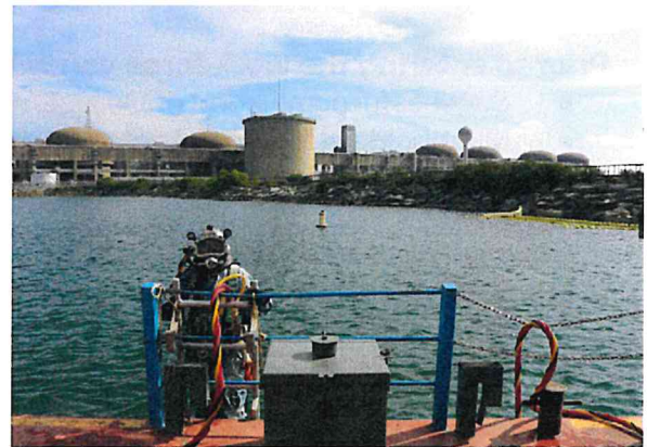
OPG Dive team finished installing a 2000 ft net around Pickering Nuclear Generating Station
